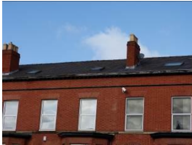
Non-conservation roof lights of different sizes disrupting the uniformity of the terraces
