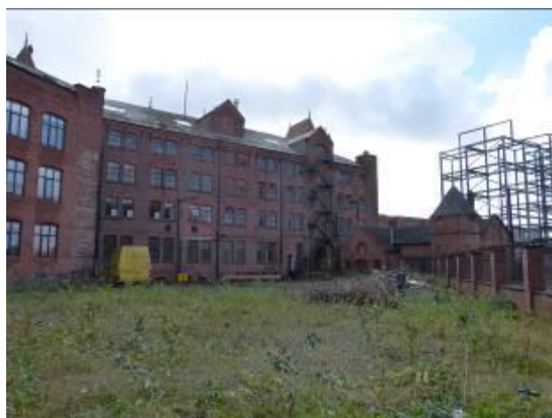
The disused open yard behind the Essence Factory, which important curtilage space
